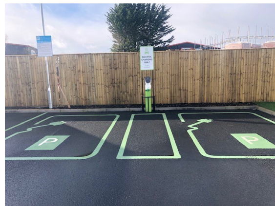
Electric vehicle charging points in a retail development
